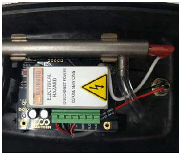
New CD cell as installed on the EOG 200
